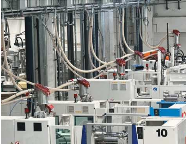
The granulate is transported inside a closed system. Feedmax Clean material loaders are also used. In this way, dust generation is reliably prevented.
