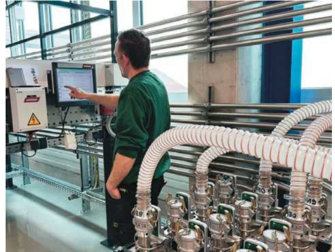
The M8 control system of the central material supply system met with a very positive response from staff members.
