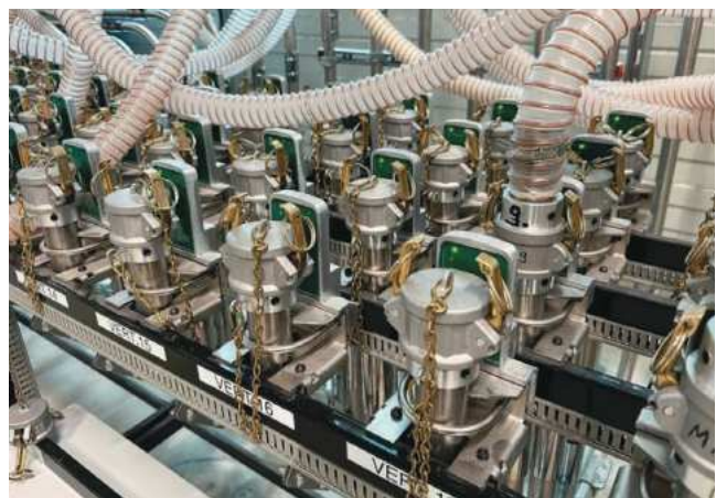
The new coupling station still leaves room for further growth.
